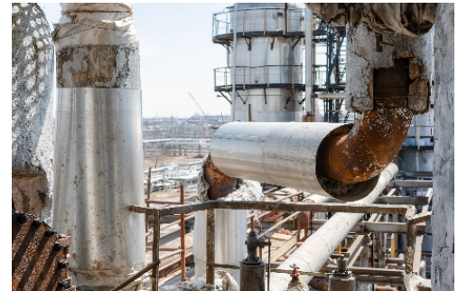
e.g., Corrosion under insulation CUI.
