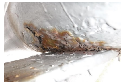
Corrosion under pipe support (CUPS).
